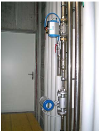
Ultrasonic flow measurement
